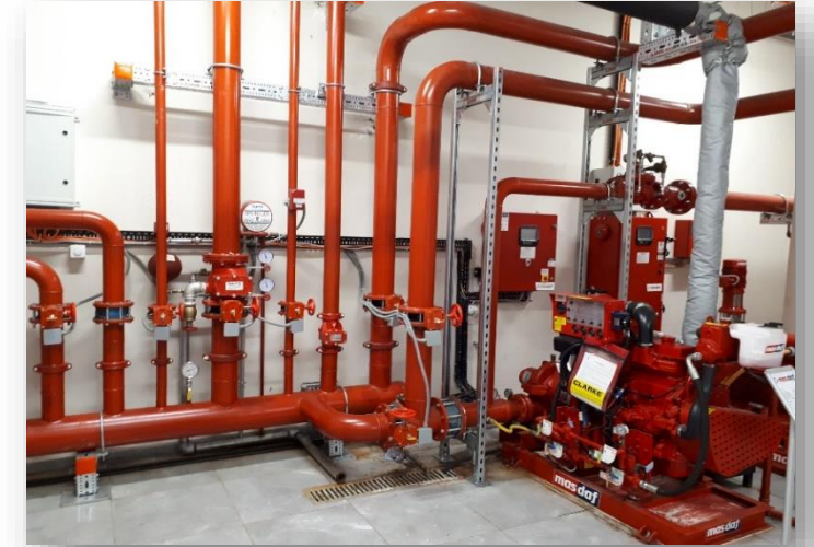
Fire Pump Station
