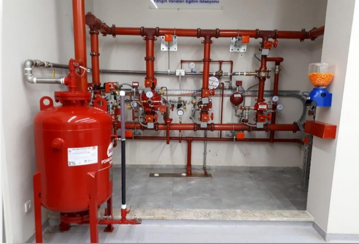
Alarm Valve Station
